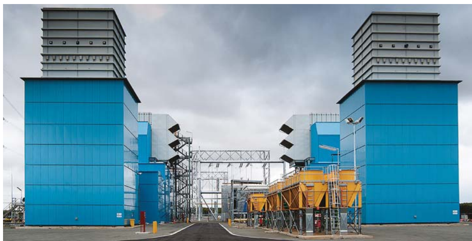
FIGURE 1.2.4 The Mortlake gas-fired power station, 200 km west of Melbourne, was opened in 2012. Natural gas from the Otway Basin is piped to this facility where it is burnt to produce electricity.
